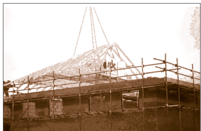
Figure 6 Roof truss built on ground and lifted into position avoiding the need to work over open joisting later on
