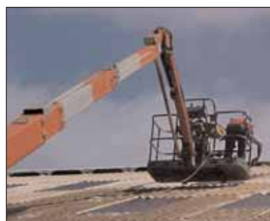
Figure 4 A mobile elevating work platform being used to replace a roof sheet
