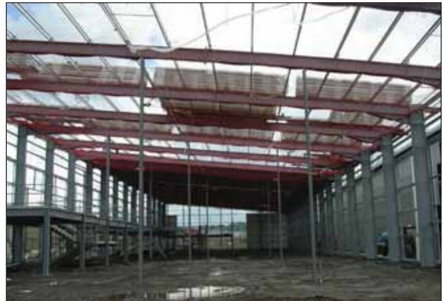
Figure 7 Safety nets installed prior to sheeting. Note that the net is fixed as close to the underside of the roof as possible to minimise the extent of any fall
